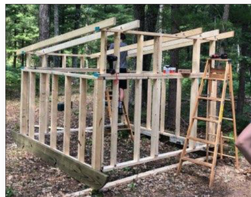
Once unloaded and the site was prepared, the walls were screwed into place.
